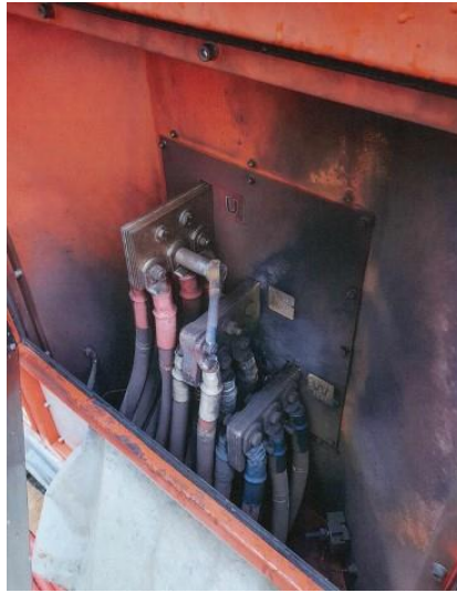
Above: Portable load bank involved in the incident
